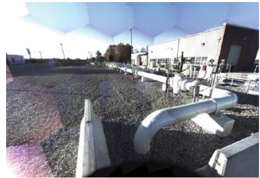
Photograph of compressor station
